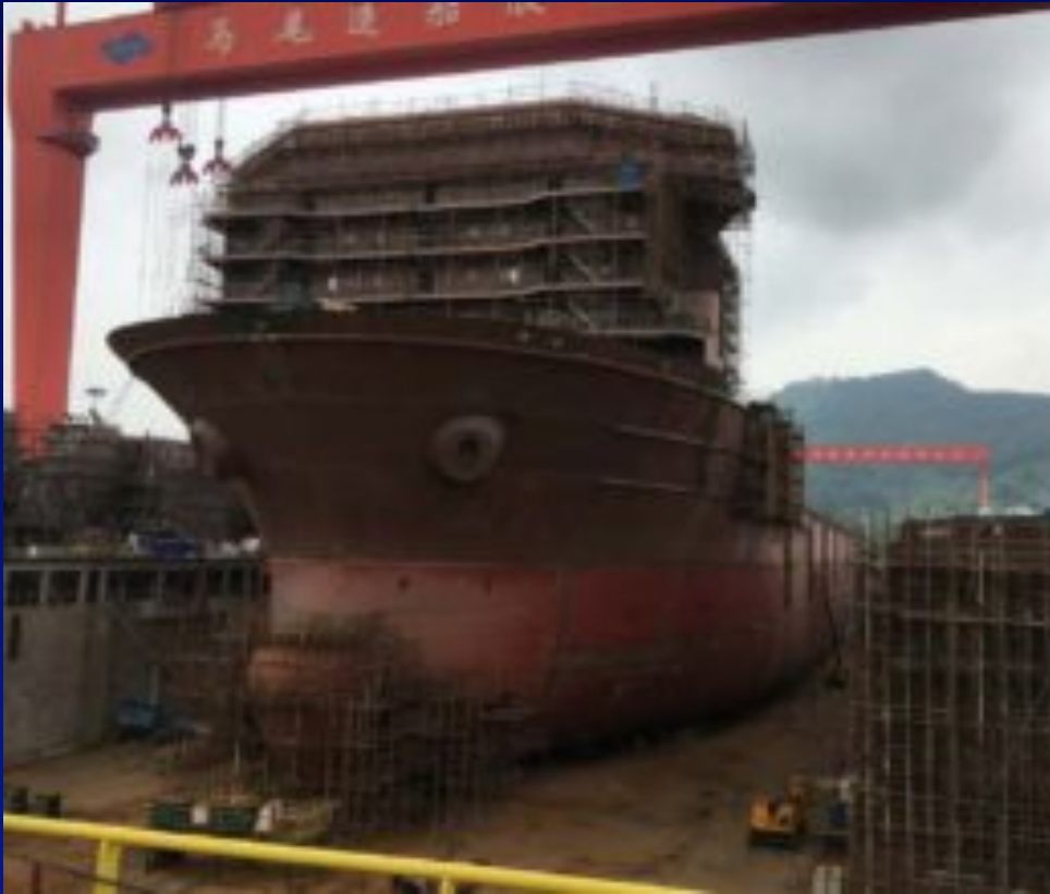
Nautilus Production Support Vessel (PSV), under construction at the Mawei shipyard in China. © Nautilus Minerals.
